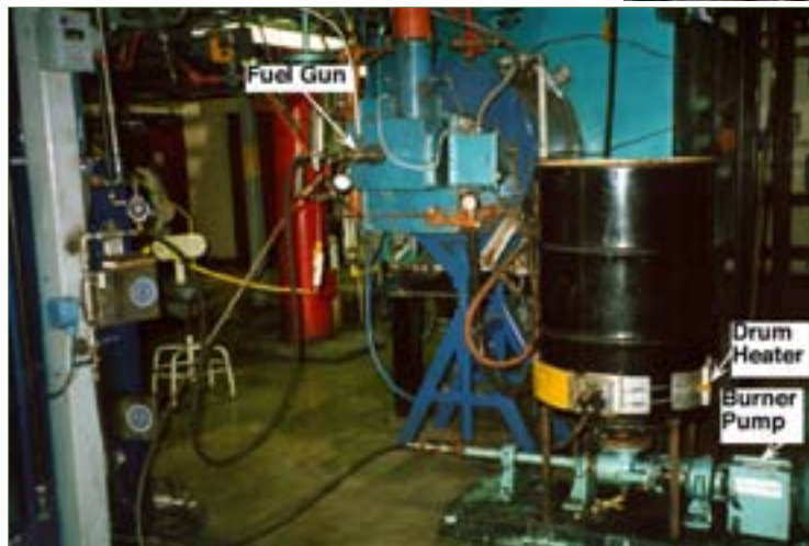
Oil-Designed Watertube Boiler Firing Lard
