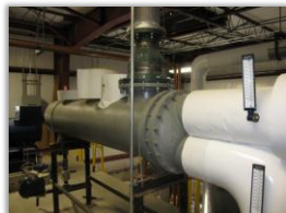
Steam to hot water heat exchanger
