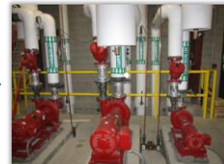
HX and Distribution Pumps to three facilities
