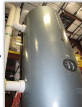
6,000 gallons thermal storage
